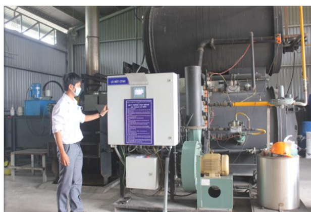
Figure 6 Hazardous waste incinerator (capacity of 200 kg/h) at Binh Duc Landfill
