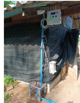
(b) Automatic Control Cabinet
