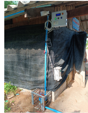
(b) Automatic Control Cabinet
