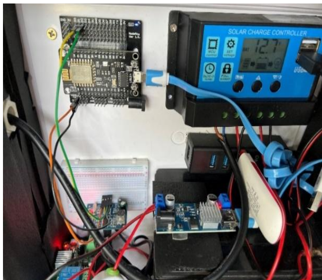
Figure 3 Hardware connection in the control cabinet.
