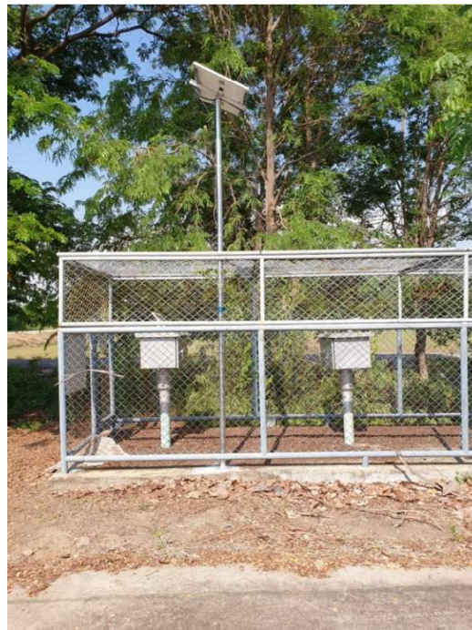
Figure 3. Installation of an automatic groundwater monitoring and recording system.
