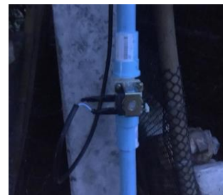
Fig. 11 Example of installing a solenoid to a water system
