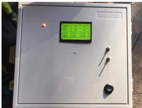
Fig. 9 The IoT control box
