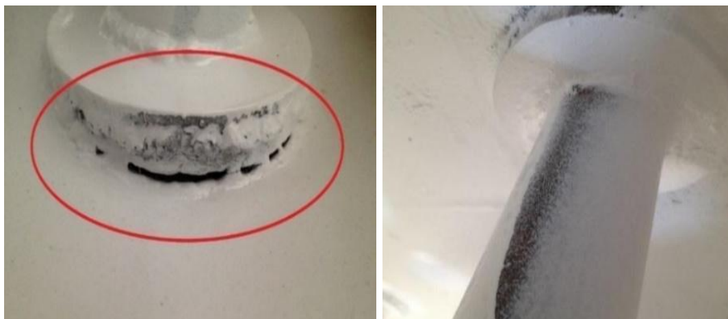
Figure 3 Defect Under the Strainer Plate
